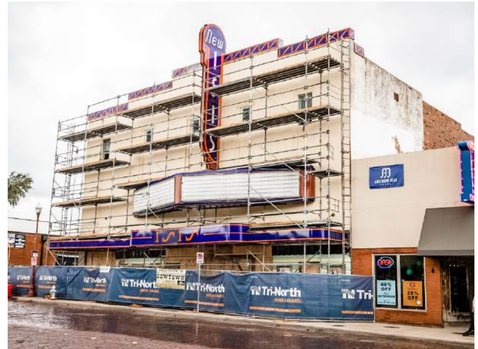
The New Isis Theater, which sat vacant for decades prior to the adoption of the Stockyards Form-Based Code, has been undergoing rehabilitation since 2018. (Source: City of Fort Worth, Development Services Department, 2021.)
