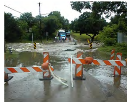
Stormwater flooding streets.
