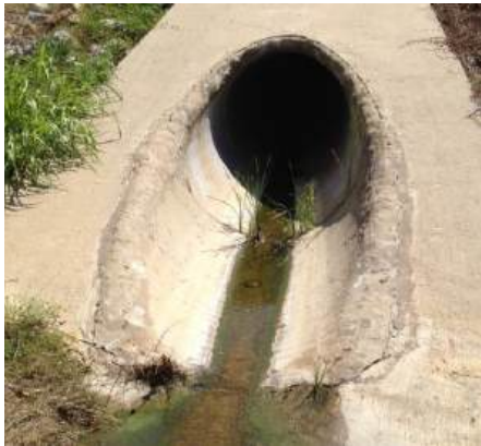
Dry weather discharge.
